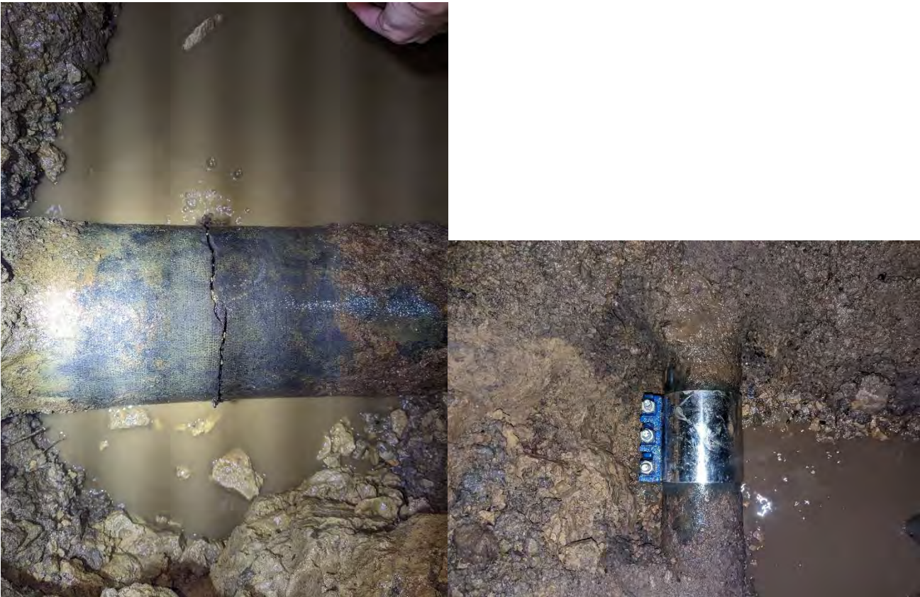
On December 22, the USW crew with the City of Galena Public works fixed a broken watermain at 720 Meeker Street.
