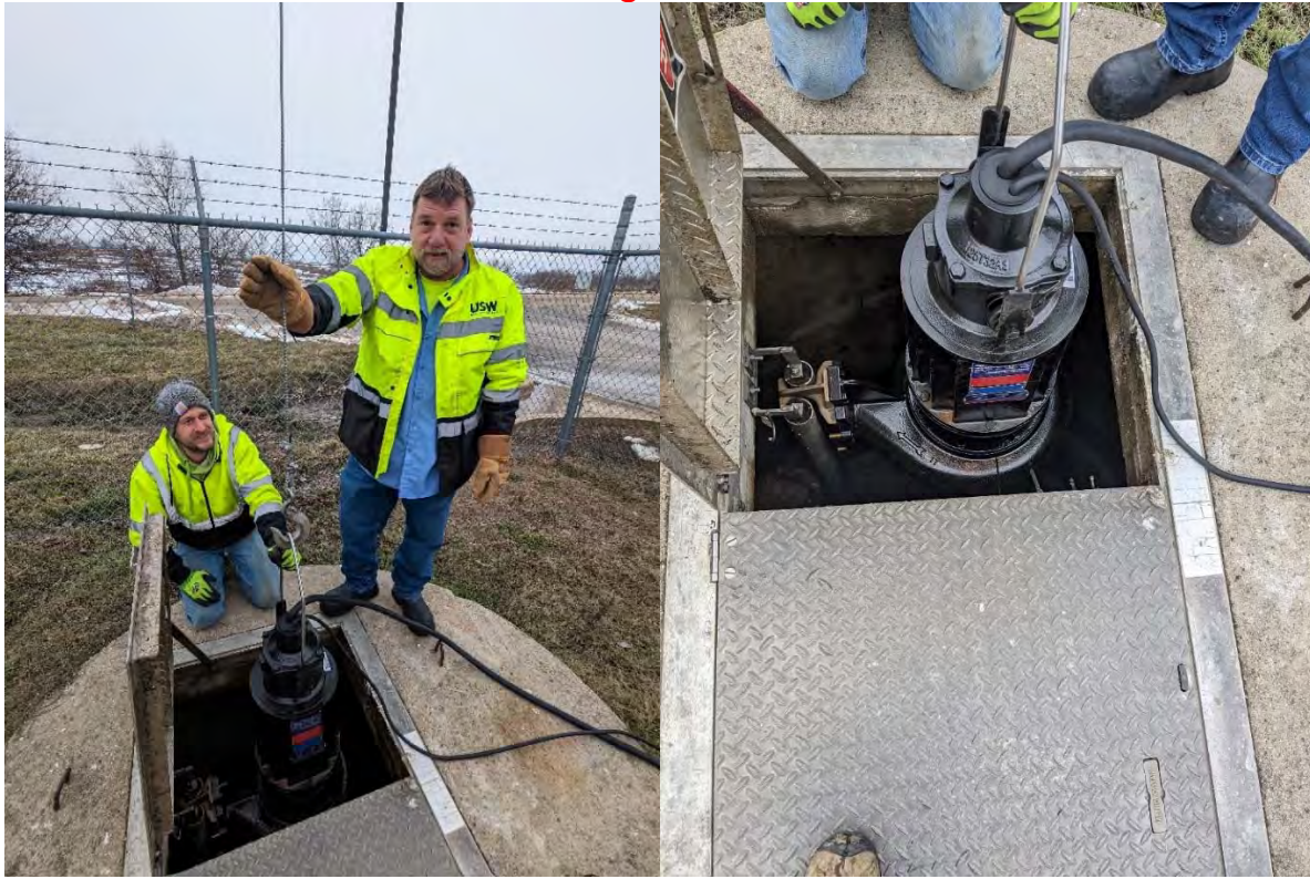
On January 31, the USW crew installed the new pump at the Hospital lift station.
