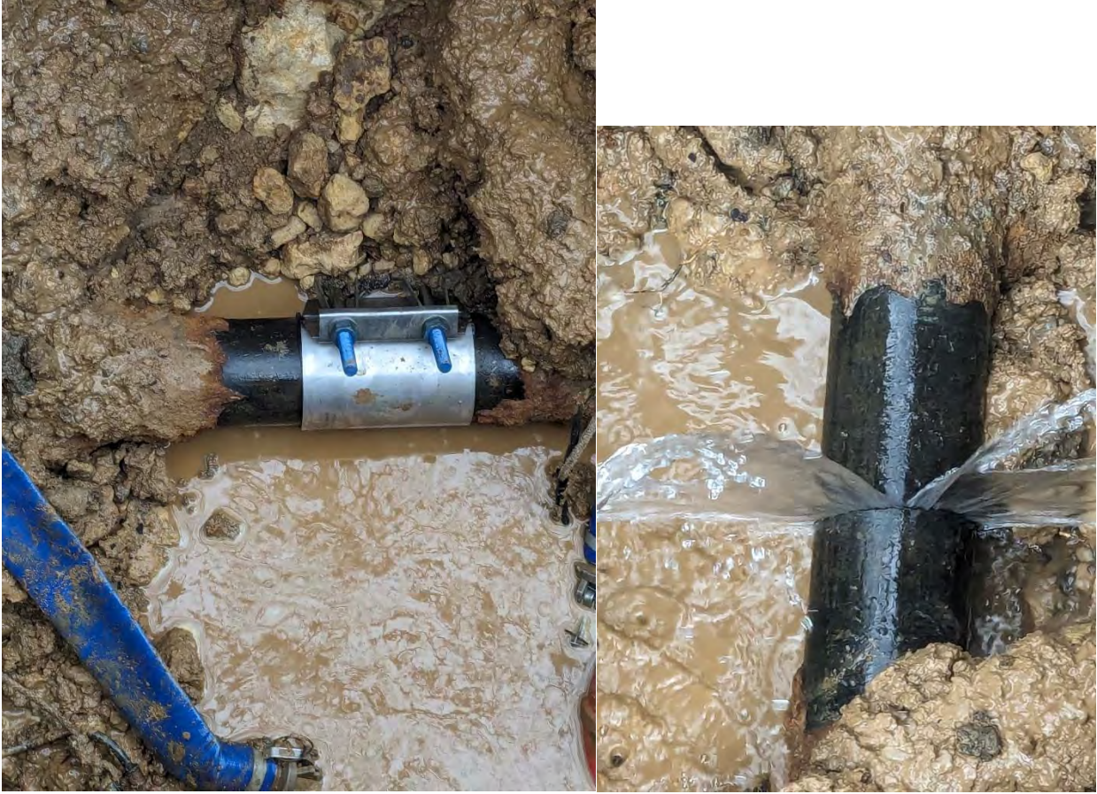
On January 11, the USW Crew and Louie's Trenching crew fixed the main at the intersection of Clay and South Hickory.
