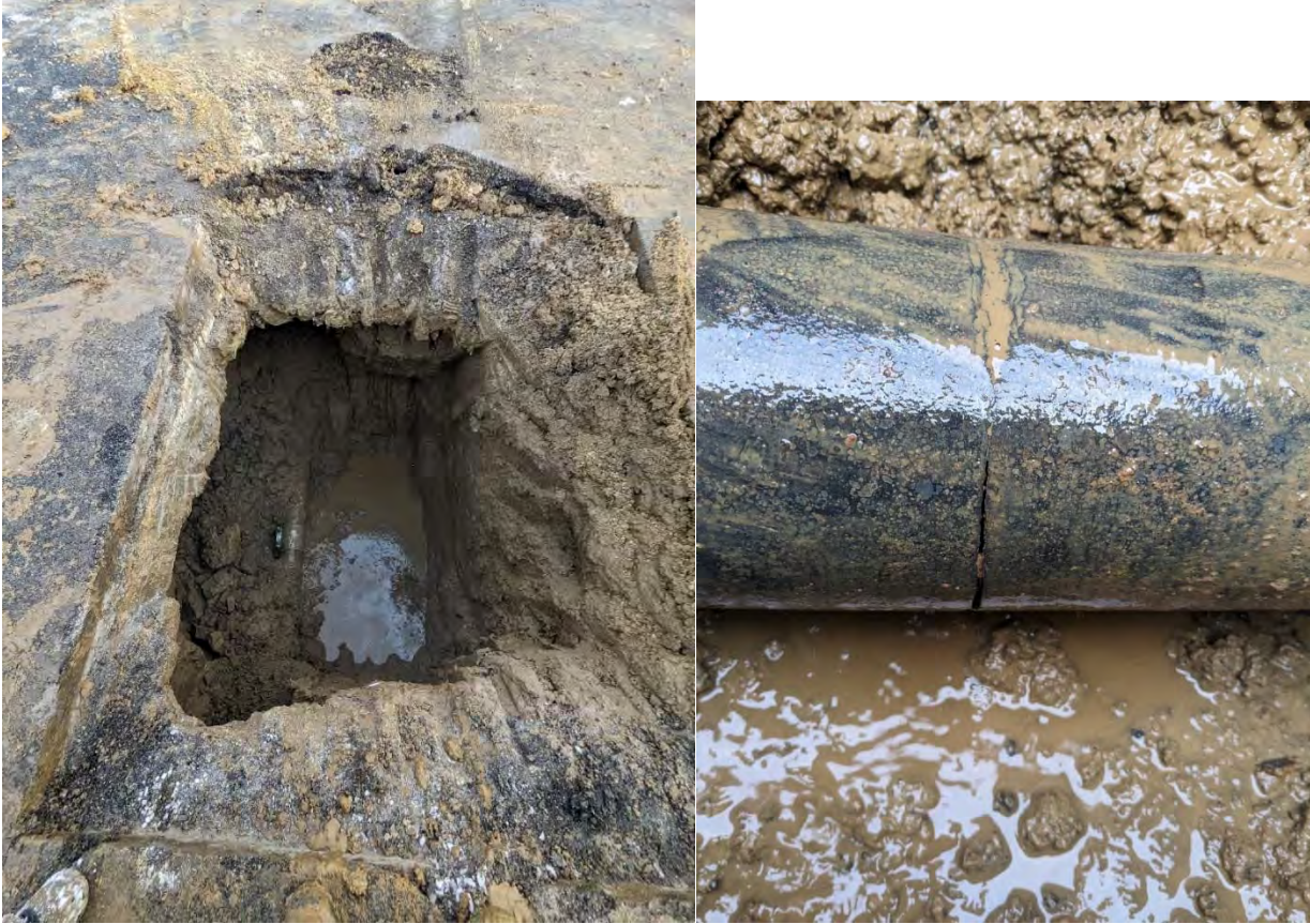
On January 19, the USW crew and Public Works fixed the water main at the intersection of 4 th and Madison Street.
