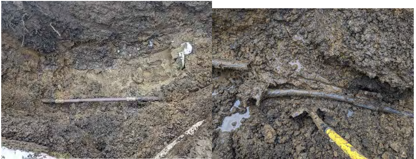
On January 22, the USW crew and Public Works fixed a 2 in. water main between South Hickory and South Division Street behind 228 Hickory St.
