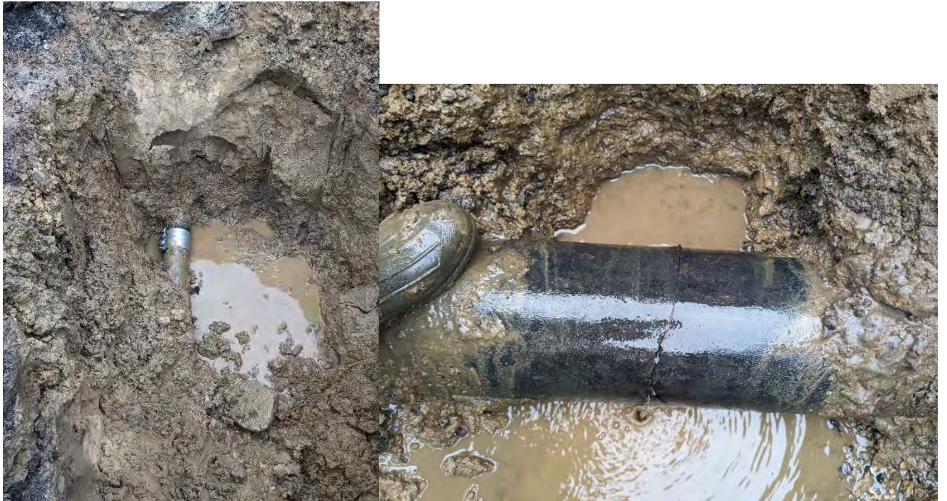
On January 3rd, the USW crew with Public Works fixed the water main in front of 605 Franklin.
