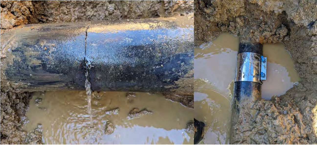
On December 12, the USW crew with the City of Galena Public works fixed broken water main at 105 Kelly Lane.
