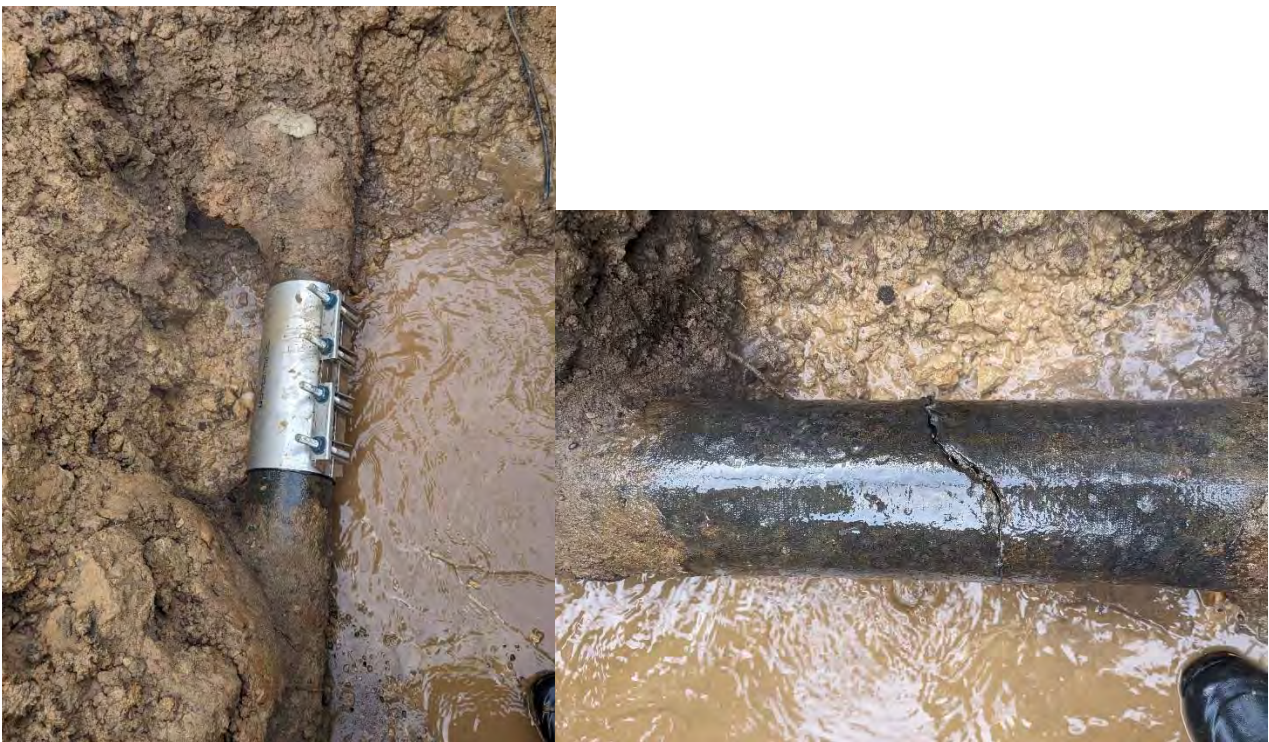
On January 13, the USW crew along with Louie's Trenching fixed the water main at 612 Washington Street.
